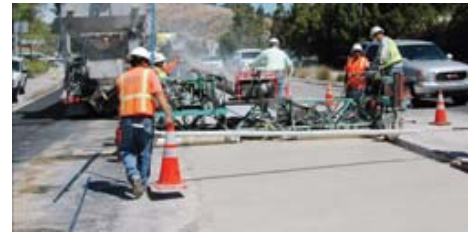
PHOTO: CTS Panel replacement work on Highway 1 in San Luis Obispo, Calif.
