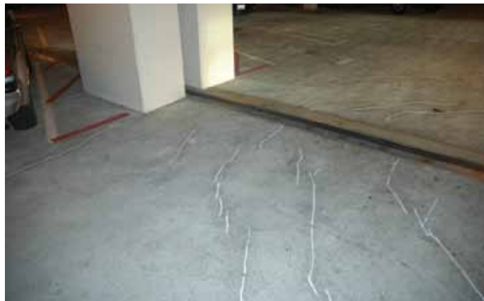
Figure 3: Top of slab near expansion joint, structure A2 Level L1.
