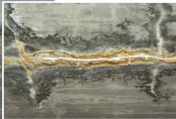
Figure 1: Efflorescence at crack on L1 slab soffit.
