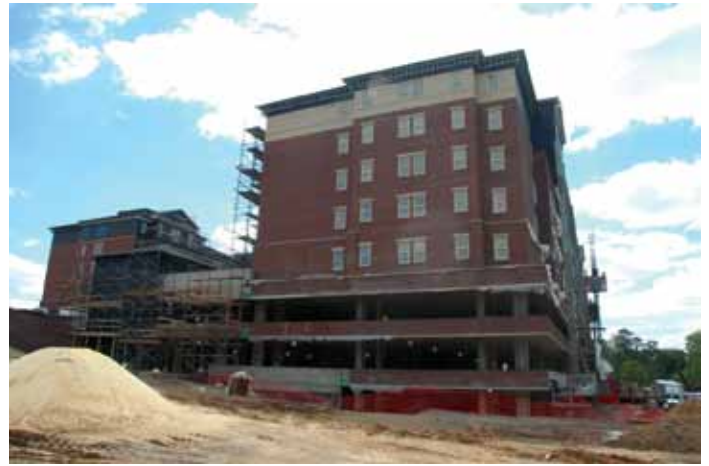
Figure 5: North elevation showing three lower parking levels and five upper residential levels.
