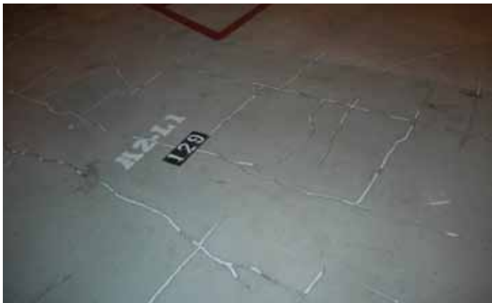
Figure 2: Typical repaired cracks on structure A2 Level L1.
